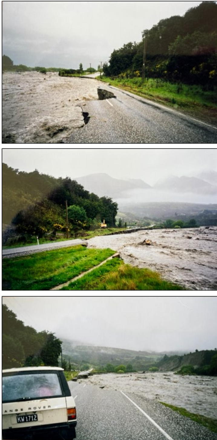
Figure 5.17 November 1999 – Buckler Burn flooding and erosion damages to the Queenstown-Glenorchy Road (photos: Kelly Family).
