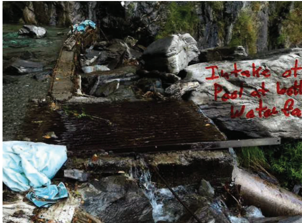
The Point of Take (screen and initial pipeline)
