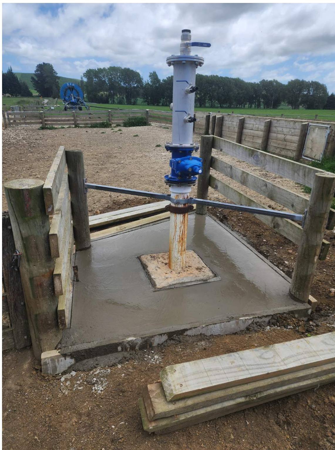
Figure 4: Upgraded headworks for monitoring artesian groundwater levels in the Papakaio aquifer in bore J41/0273. The assembly will be enclosed in a lockable cabinet. Photo provided by Nick Boyens.
