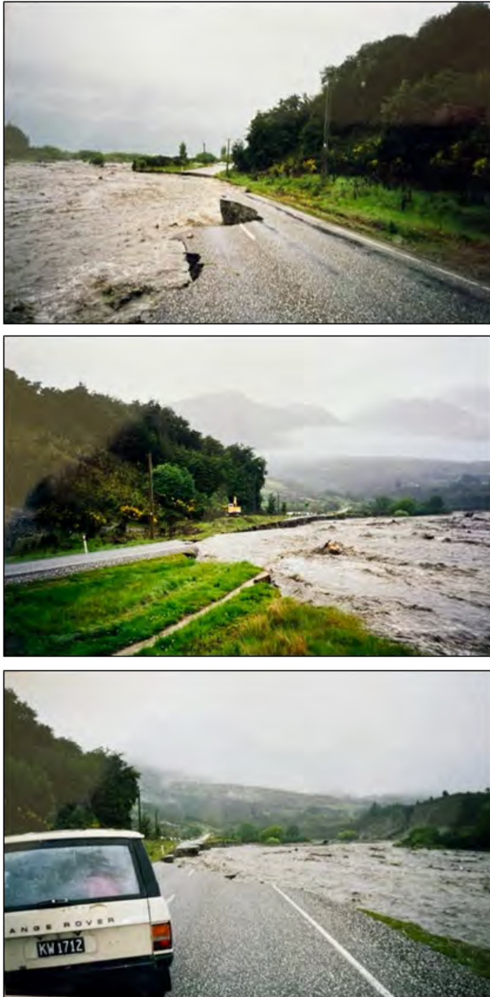
Figure 5.17 November 1999 – Buckler Burn flooding and erosion damages to the Queenstown–Glenorchy Road (photos: Kelly Family).
