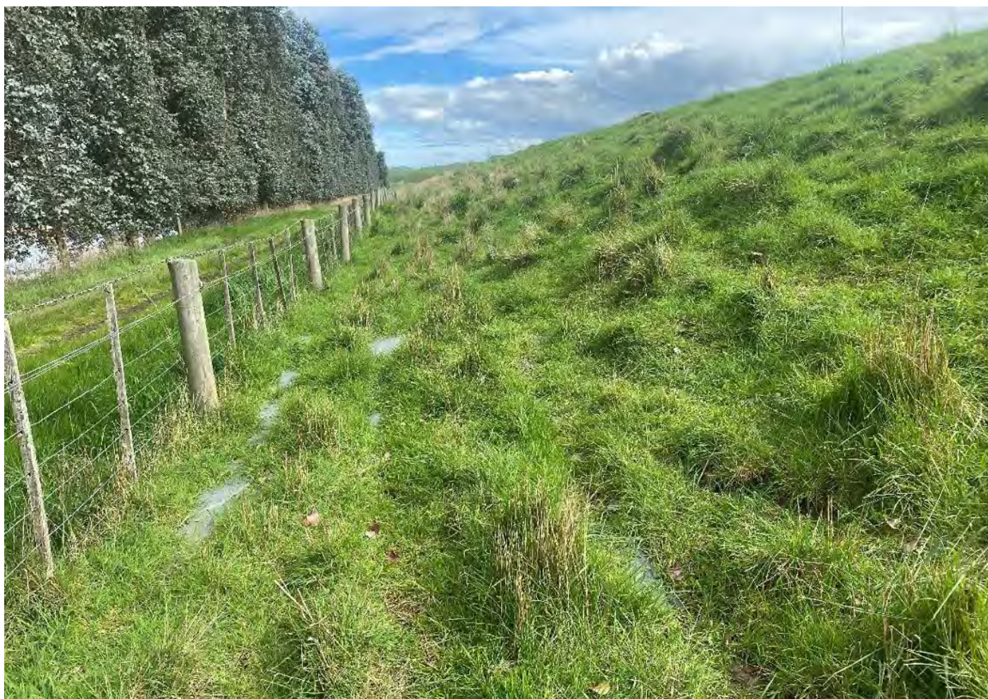
Figure A-5: Puerua River left floodbank piping.
