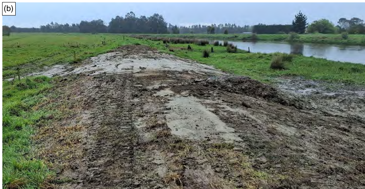
Figure A-3: Puerua River floodbank (a) cut to relieve interior flooding and (b) after temporary repair.
