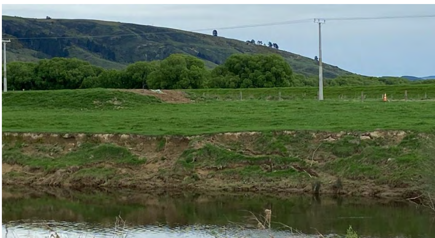
Figure A-6: Taieri River right bank berm erosion and slumping.
