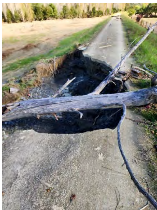
Figure 2: Post Cyclone Gabrielle Hawkes Bay showing a damaged stop bank with a SUP
