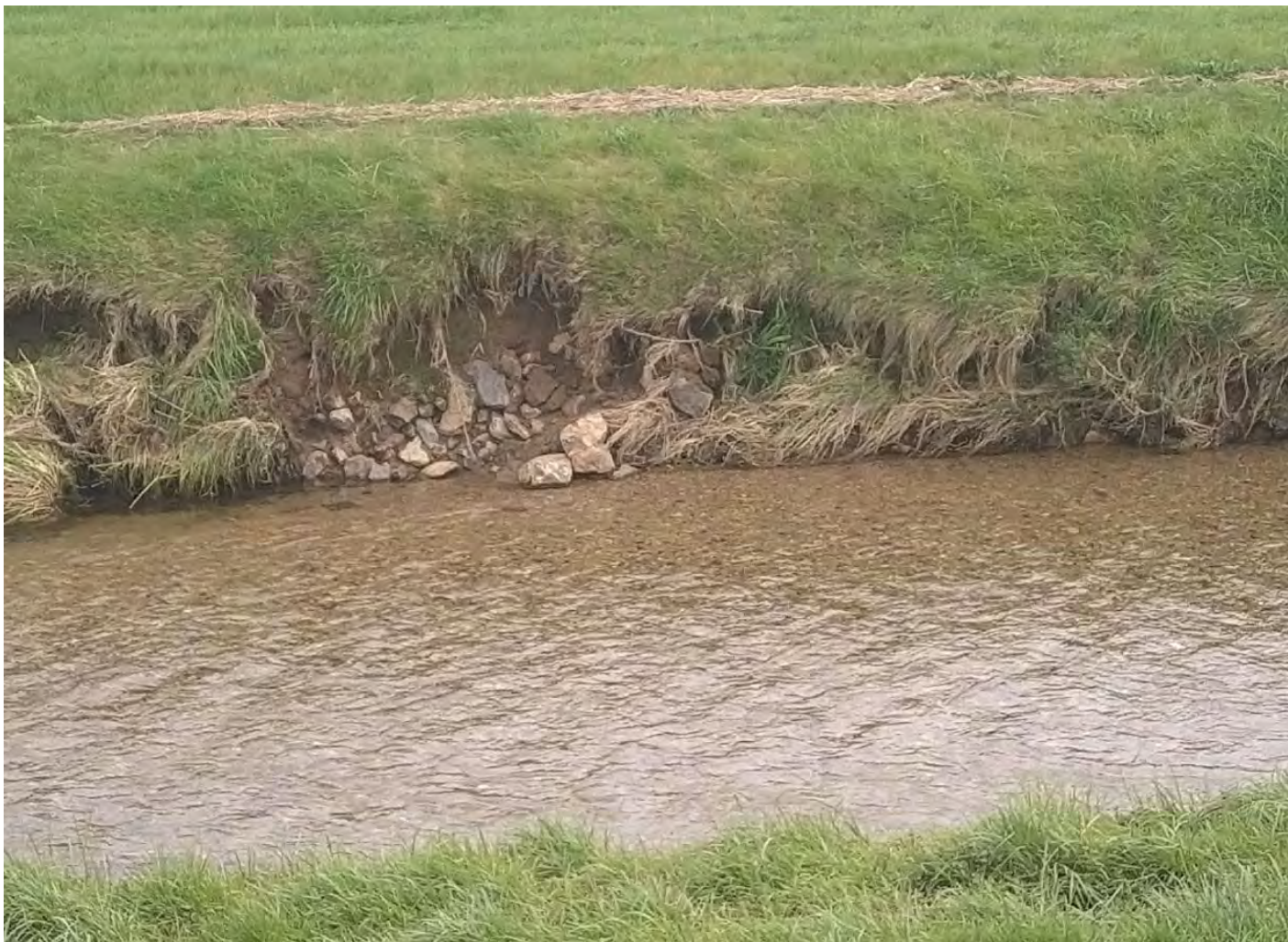
Figure A-8: Silver stream at Gordon Rd spillway showing bank erosion and high water debris line.
