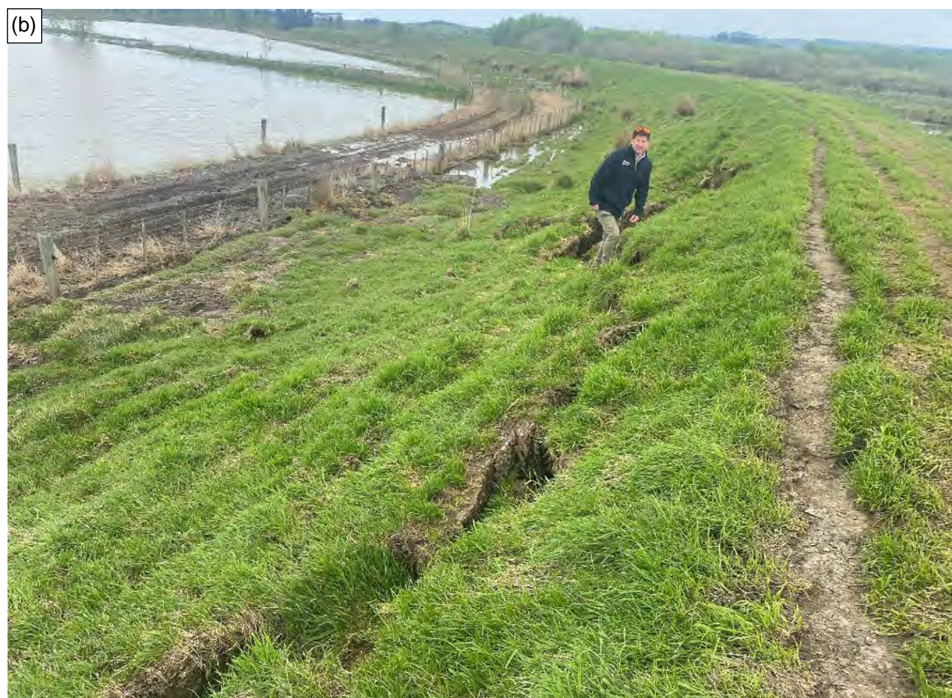
Figure A-4: Puerua River left floodbank slump downstream of Owaka Highway (a) looking upstream and (b) looking downstream.
