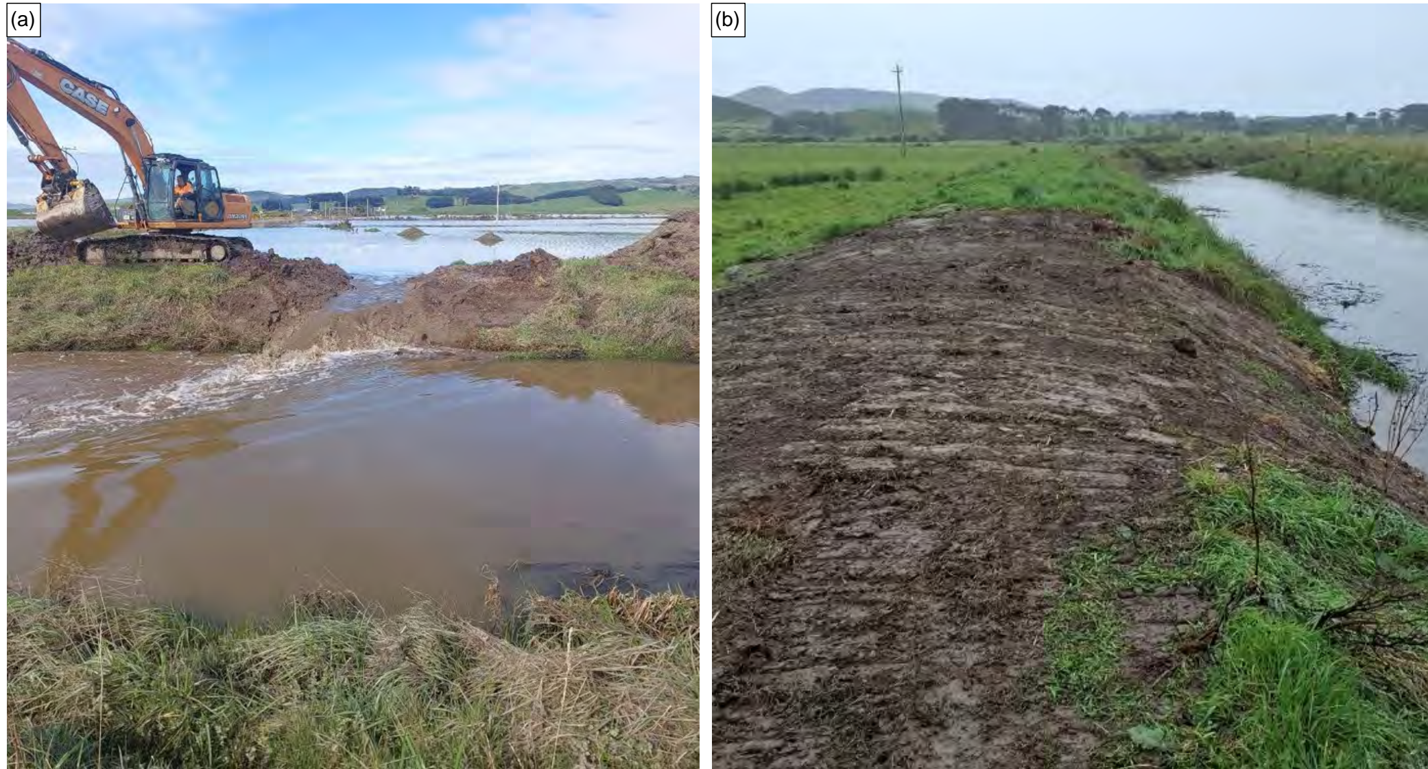
Figure A-2: Barrata Creek floodbank Puerua (a) cut to relieve interior flooding and (b) after temporary repair.
