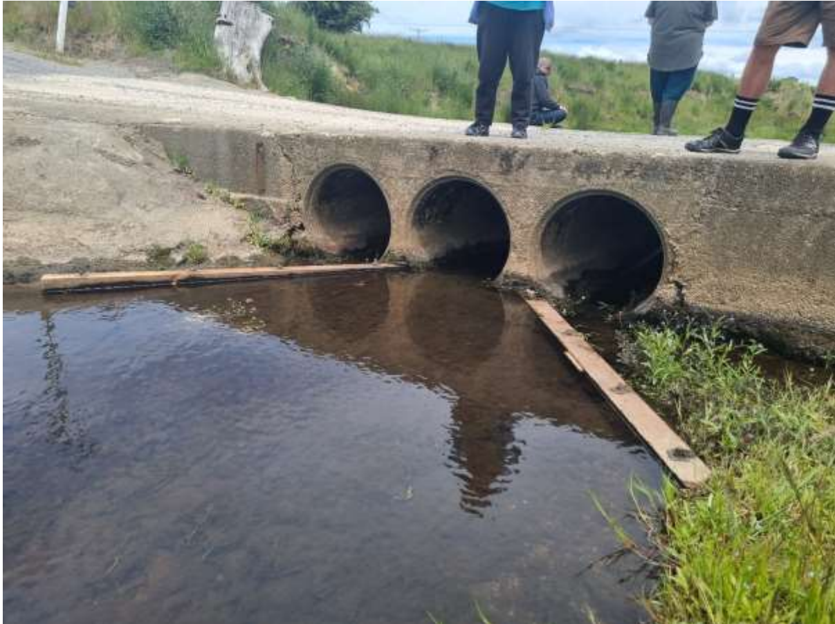
Figure 50 Upstream view of the H4 ford at Pattersons Rd showing wooden baffles to channel flows into the central culvert.
