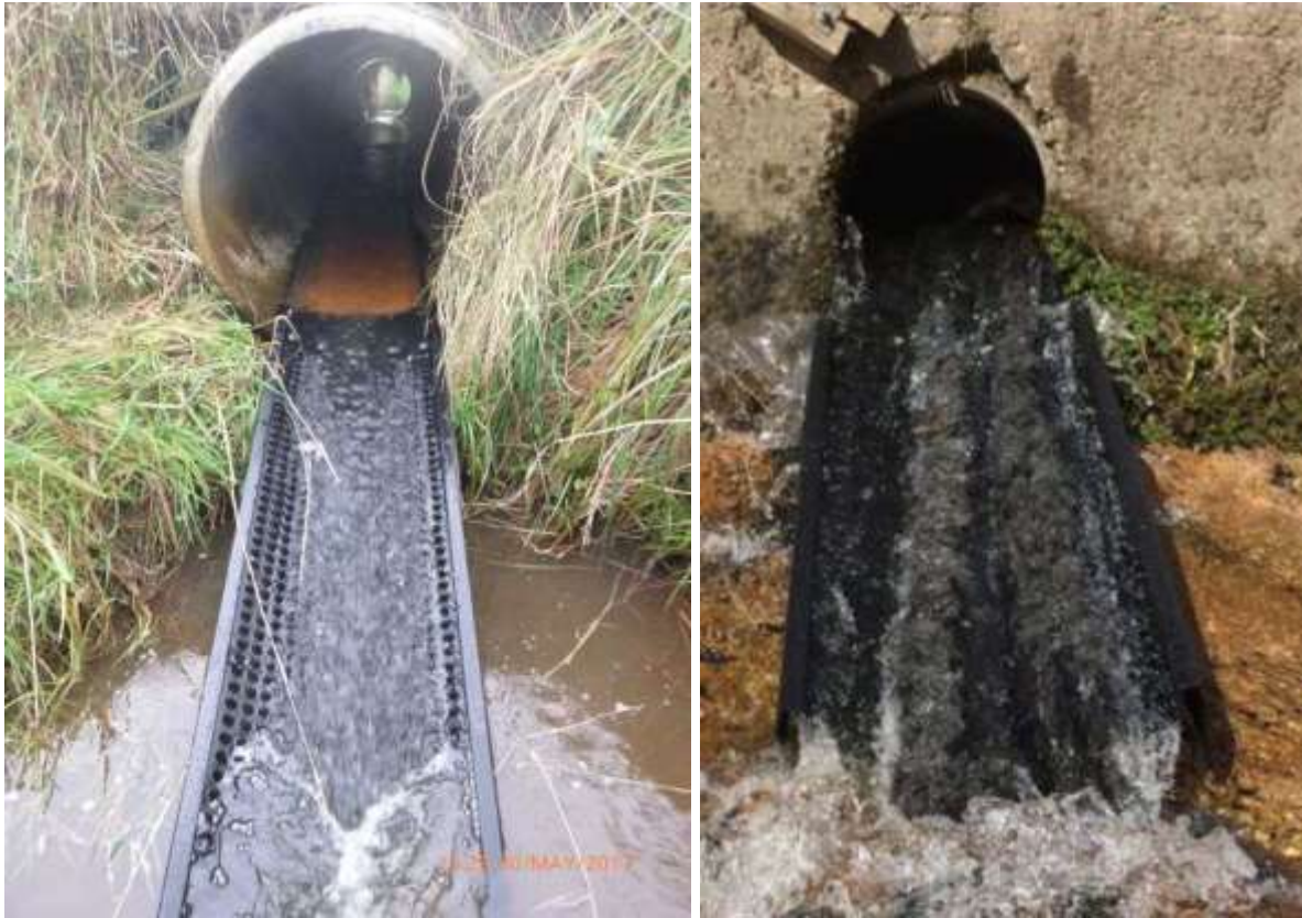
Figure 6 Examples of the retrofitting of floating ramps to existing culverts. The ramp on the right also includes mussel spat ropes to further improve fish passage.
