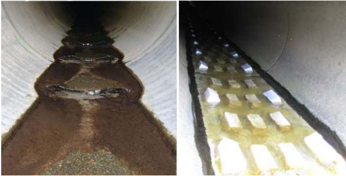
Figure 7 Examples of the retrofitting of in-culvert baffles to reduce water velocity through existing culverts
