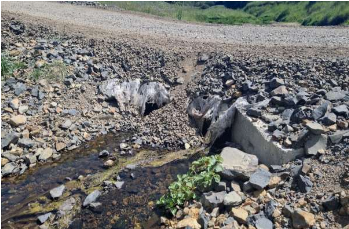
Figure 44 Partially collapsed ford preventing fish passage at the H2 site on December 7 th , 2023.
