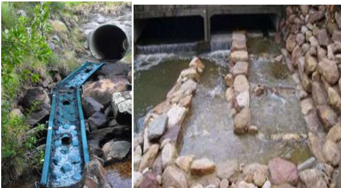
Figure 5 Example of the retrofitting of a rock ramp to an existing culvert
