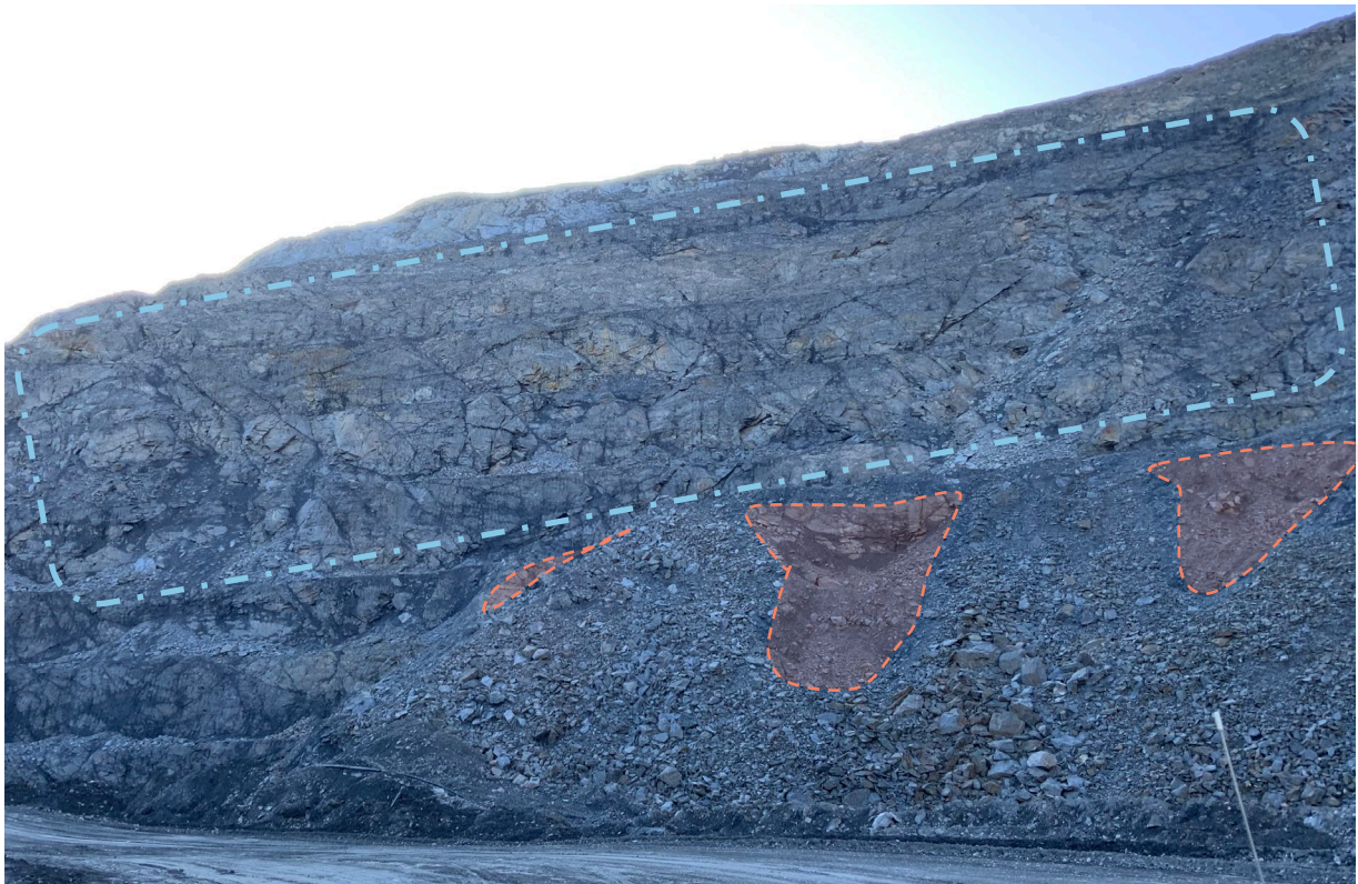
Photo 8: Fraser 6/FRIM north wall - Surface caving expression of near surface stopes highlighted in orange. Dilated structures associated with rock mass relation visible through the zone in blue.
