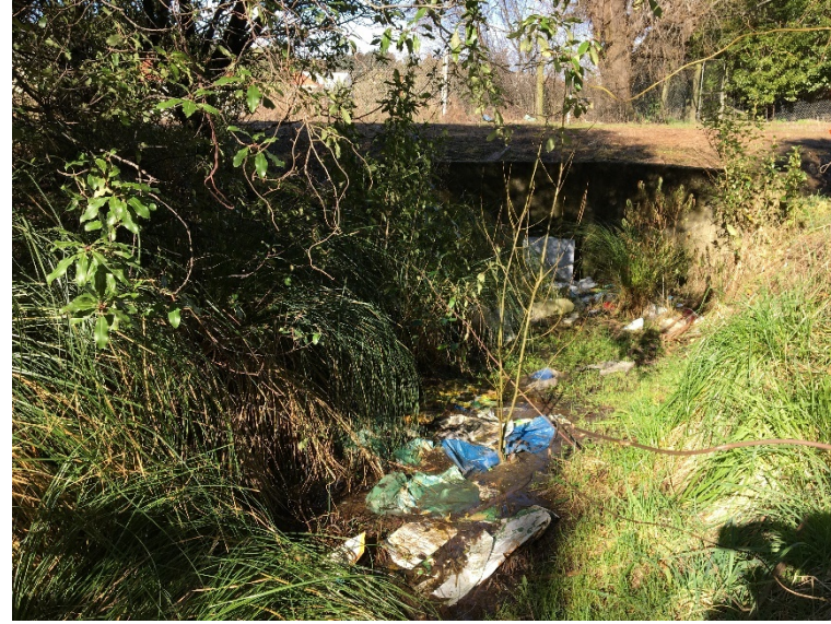
Figure 27: Culvert inflow to the constructed wetland from Taylor Street. Image taken 11 th August 2021.
