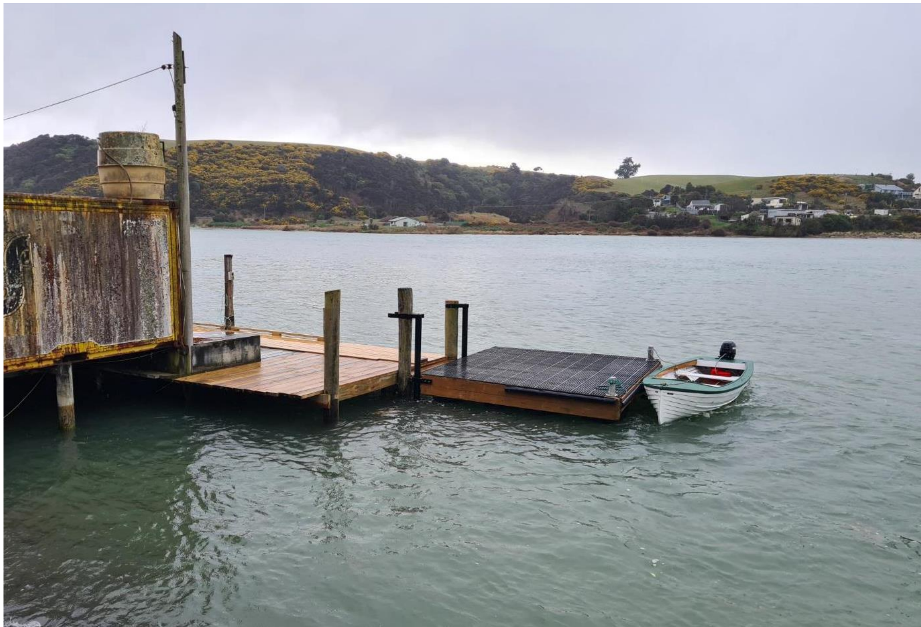
Wharf repairs and recovered/repared floating pontoon – provides all tide access to the wharf
