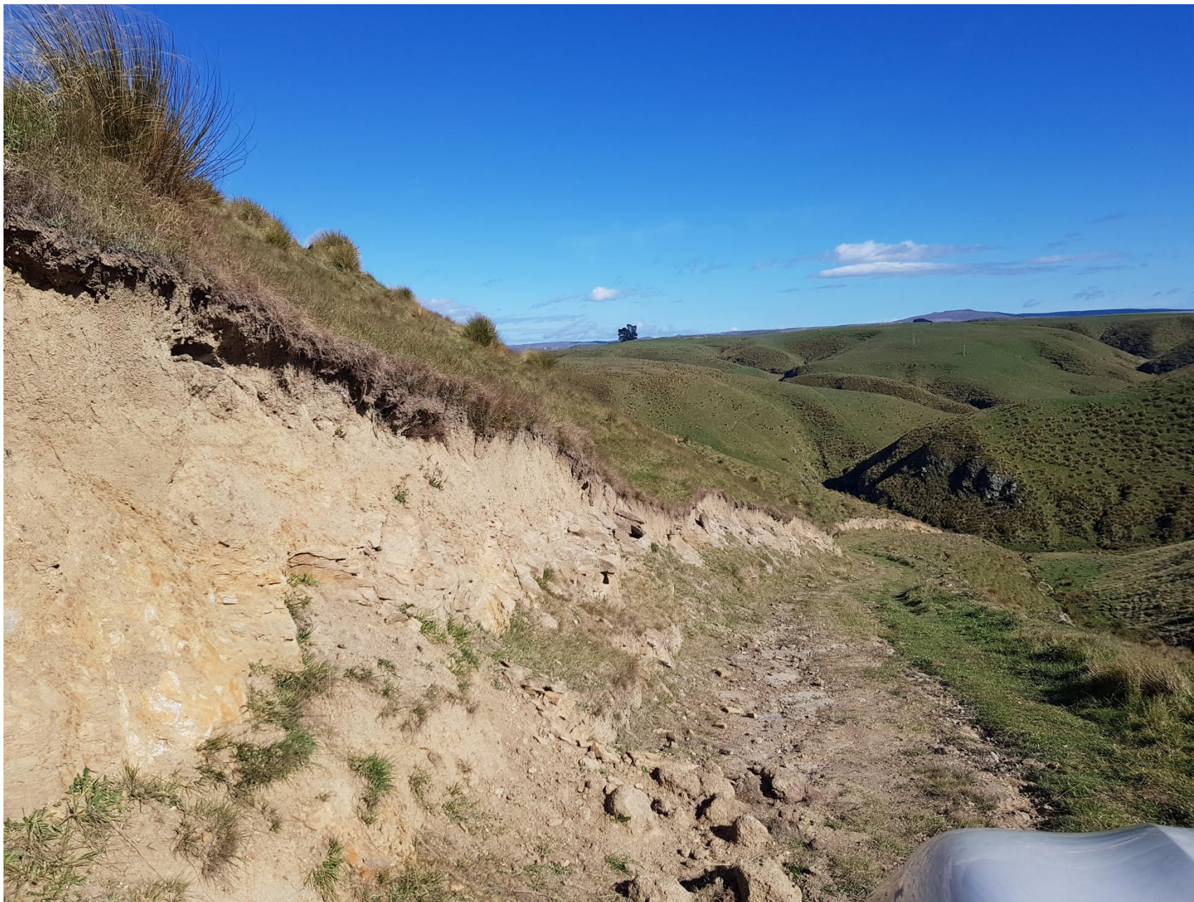
Photo 5: Exposure of loess soils over schist in access track cut down to Clydesdale Silt Pond
