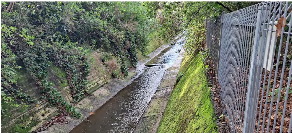
Figure 2. Typical sections of the Lindsay Creek channel in North East Valley (all looking upstream). Note the narrowness of the channel, the steepness of the right bank and the proximity of the houses and residential activities at many locations along the stream channel. The concrete channel lining and floodwall are ORC assets, some infrastructure is also owned, controlled and maintained by Dunedin City Council and adjacent private landowners.
