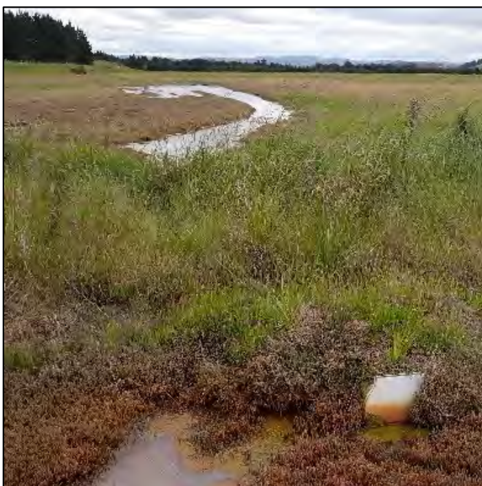
Drainage pipe with flap gate blocking tidal inundation with herbaceous saline vegetation in the background.
