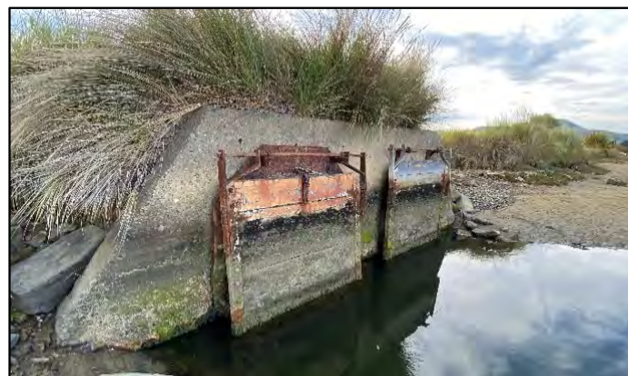
Flap gates on culverts prevent tidal inundation.
