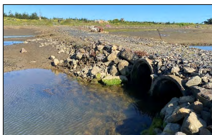
Causeway, with recently (last 5 years) installed culverts restricting tidal inundation in East Arm.
