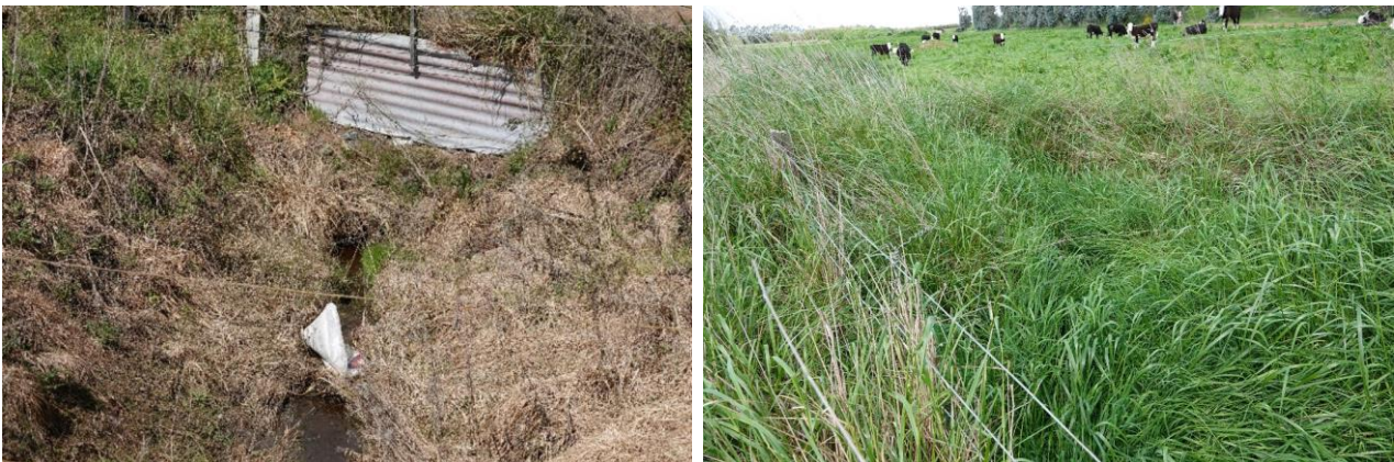
Figure 7: Culvert inlet (left) and drain on the other side of Kaitangata Highway (right). 4 November 2022.
