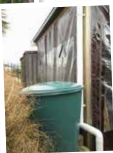
Water tank installed
