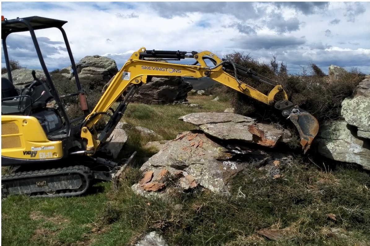
Figure 5.3. Machine-assisted dismantling of a rock tors during the Deepdell North III Project. Image by M. Tocher.
