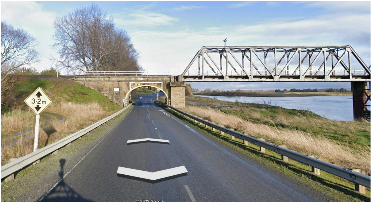
Figure 2 Railway overbridge Height Restriction
