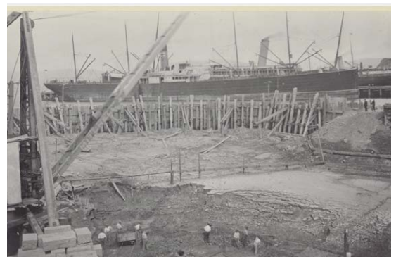
Figure 46 Elevated view of men excavating seabed soil at Port Chalmers (1907). Credit: Hocken Digital Collections
