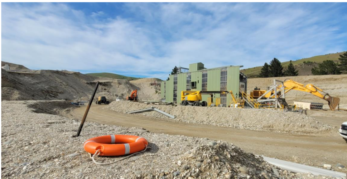
Figure 5. Floating gold processing plant currently being constructed at the base of the test pit.
