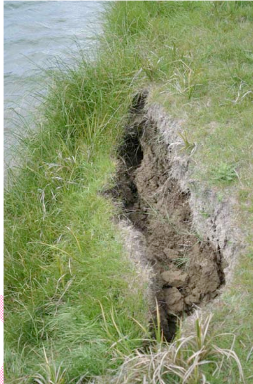
Figure 2. Bank erosion along the true right bank of the Kakanui River Estuary.
