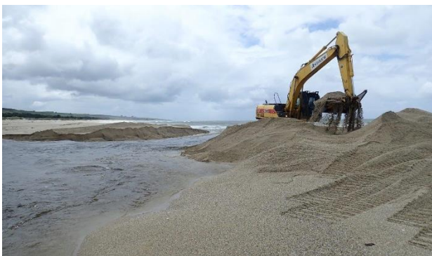
A digger was opening the Toko Mouth at the time of the 2020 survey. It had been fully closed prior for a period of ~10 days.
