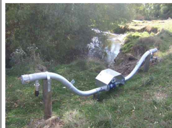
Meter location alongside Lauder Creek Source: ORC Inspection Sheets
