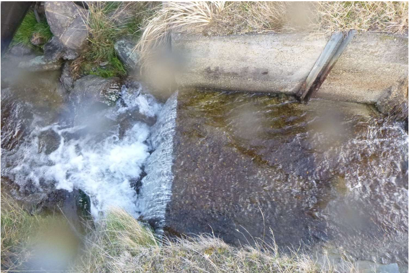
Figure 17 Photograph of the County race intake on Coal Creek from the True Right bank.
