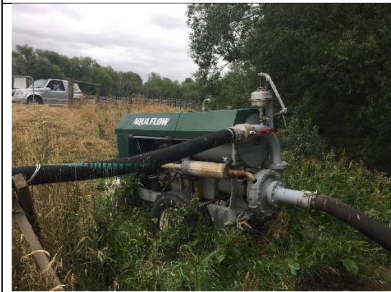
Pump set up at intake Source: ORC Inspection Sheets
