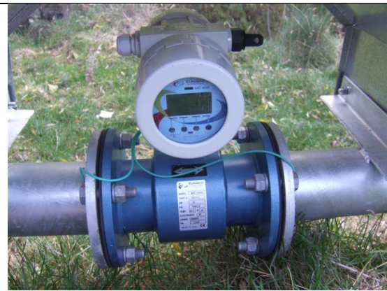
Meter Source: ORC Inspection Sheets
