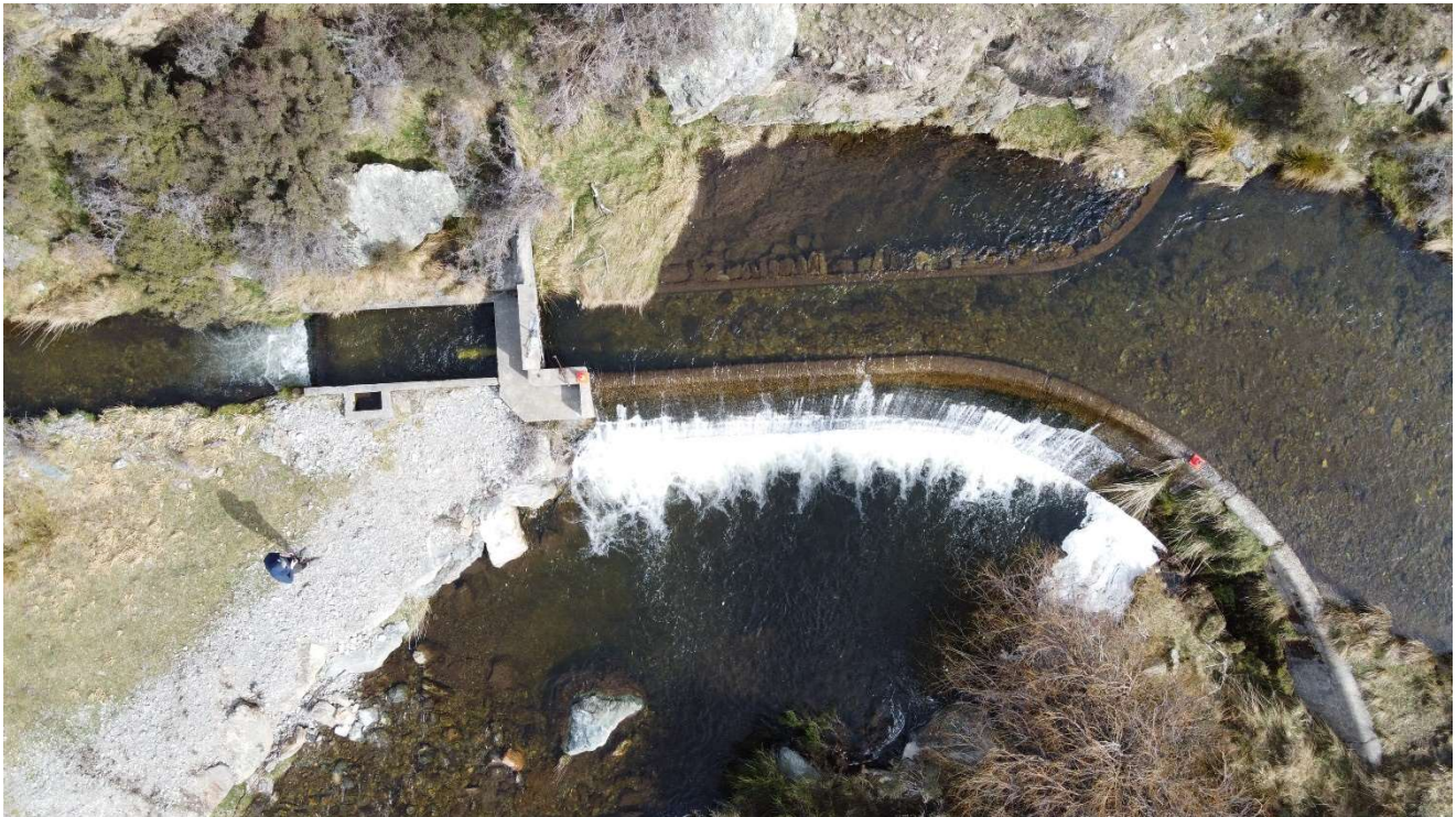
Figure 12 Aerial photograph of the Matakanui race intake on Thomsons Creek.
