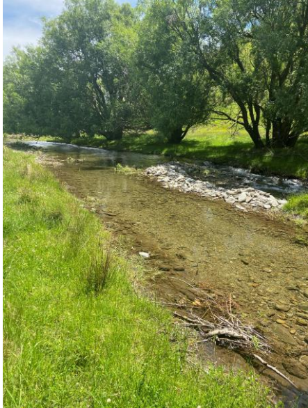
Permit 94548 Intake location consisting of gravel and rock bund guiding the flow to the intake race
