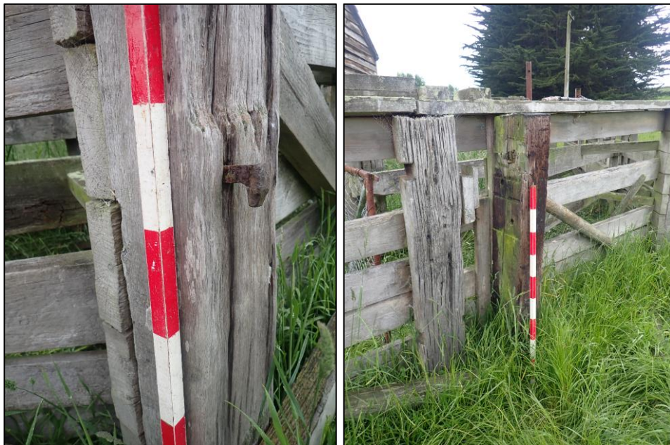
Figure 7-11. Repurposed railway sleepers with iron spikes, utilised in the construction of the yards.
